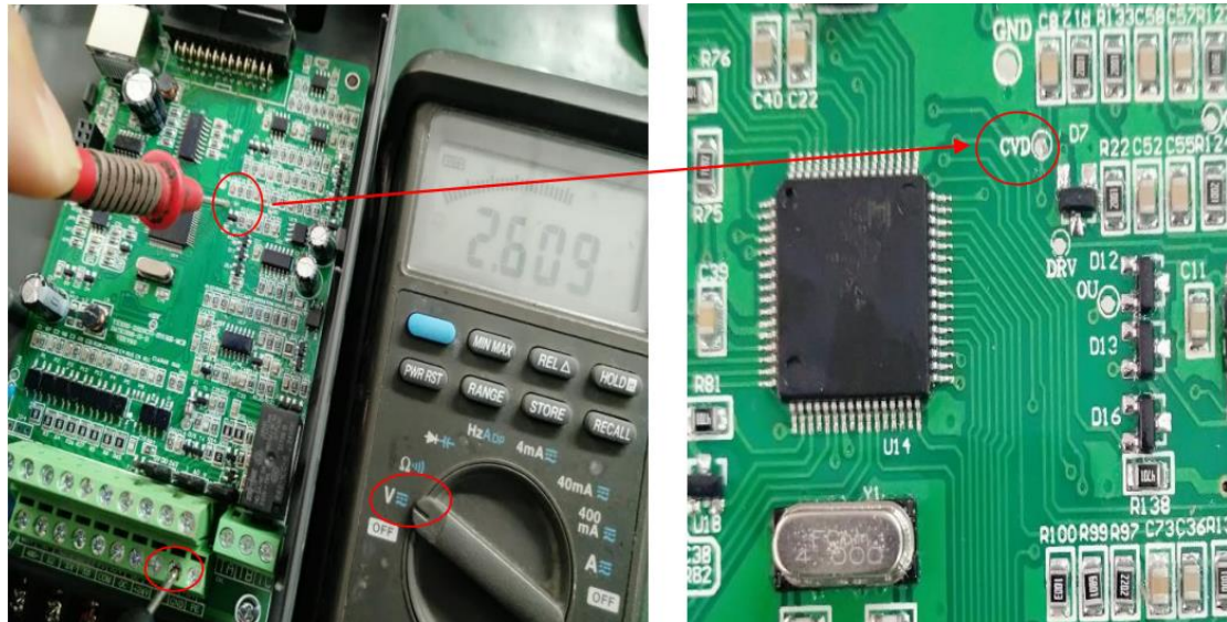
Figure. 10 Black Probe Placed on the GND Terminal of the Control Board, and Red Probe Placed on the CVD Point
